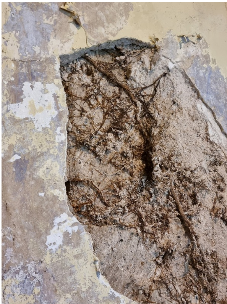
Ivy roots under the plaster and through the paint layers
