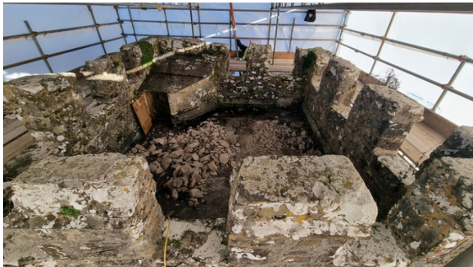
Churches never fail to surprise: the 1950s concrete roof on the tower was, we discovered, reinforced with an iron bed-frame!
